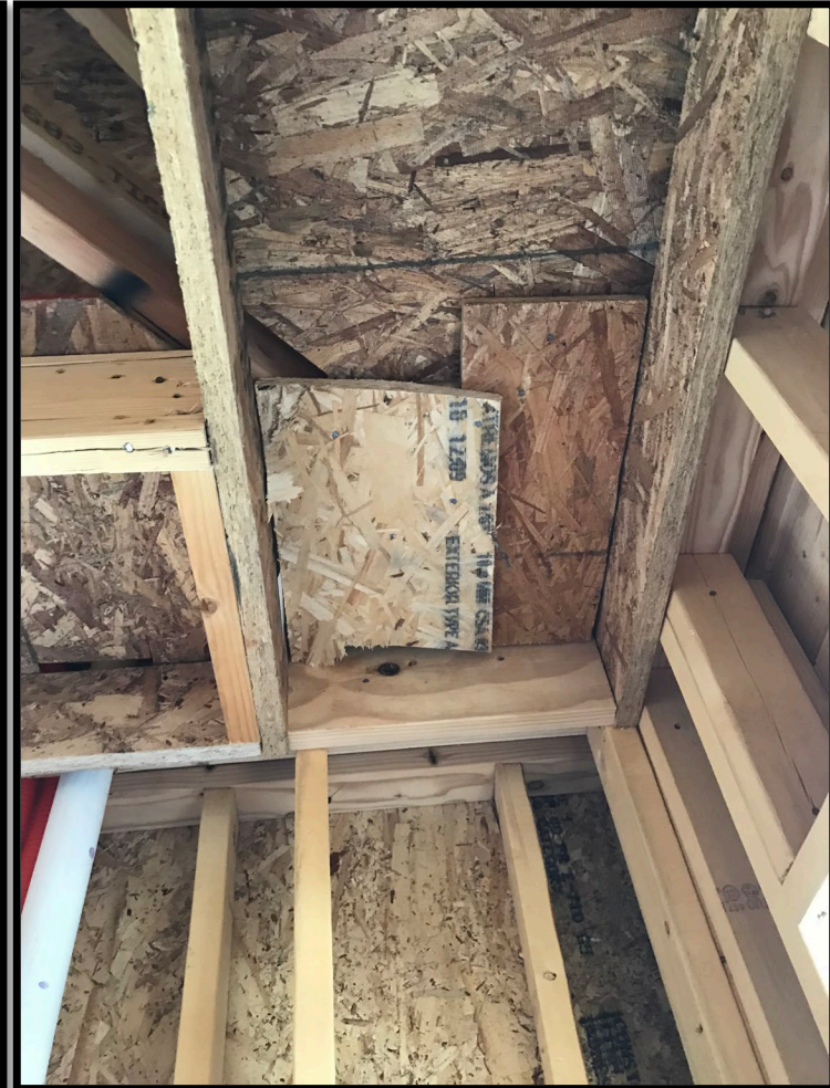
Holes in Materials & No Sealant
