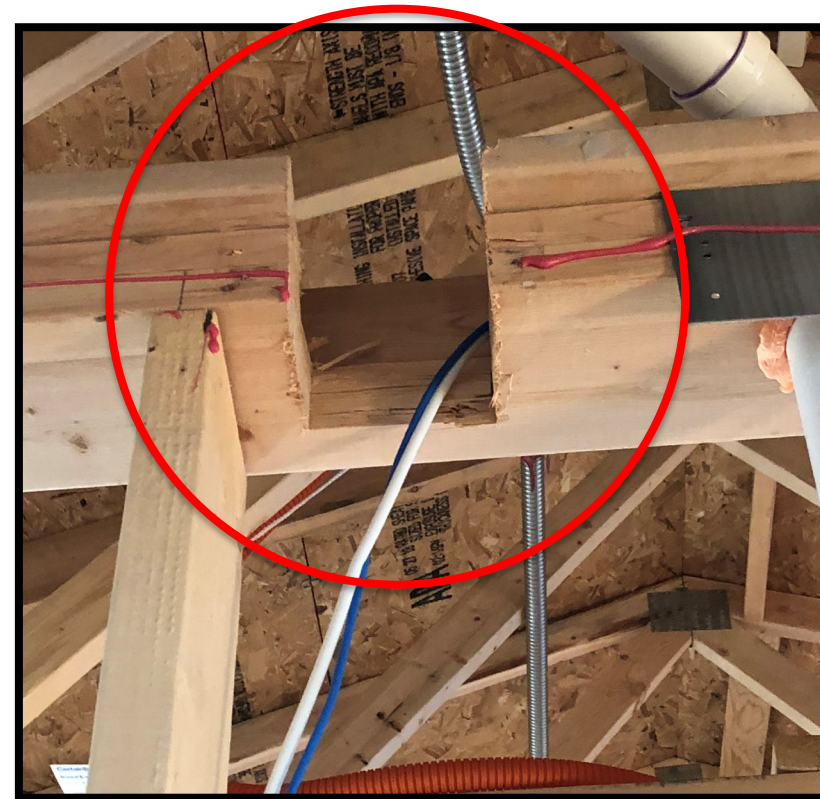
Large Hole Can't Be Sealed
