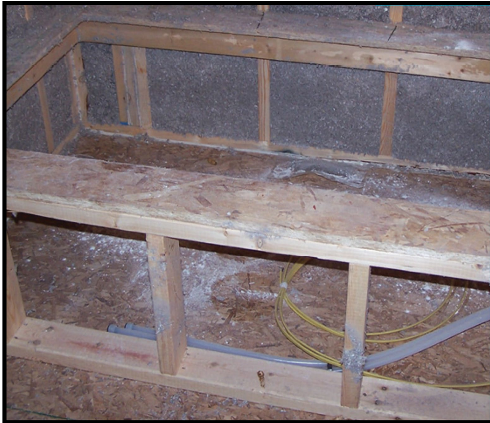
Insulation installed behind tub enclosure needs an air barrier prior to tub install
